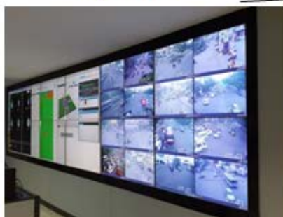
Surveillance Camera Control Room
